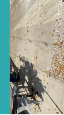
Deteriorating sidewalk pavement
